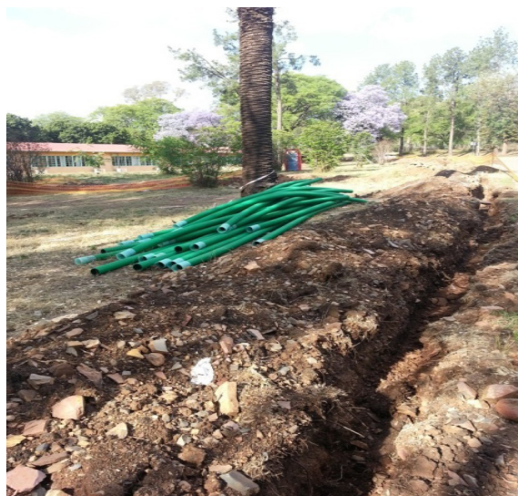
Weskoppies Hospital: Emergency power upgrade and street lighting
