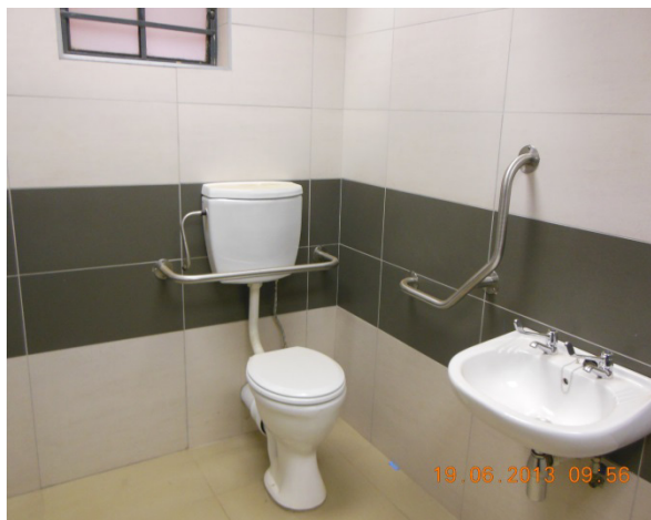
Chief Albert Luthuli School: Disabled Toilet Facilities
